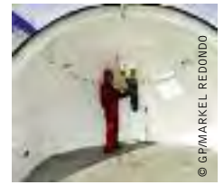
image A WORKER ASSEMBLES WIND TURBINE ROTORS AT GANSU JINFENG WIND POWER EQUIPMENT CO. LTD. IN JIUQUAN, GANSU PROVINCE, CHINA.
