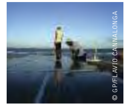
image CHECKING THE SOLAR PANELS ON TOP OF THE GREENPEACE POSITIVE ENERGY TRUCK IN BRAZIL.
